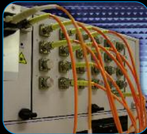
Fiber Optic: Single and multimode testing.
